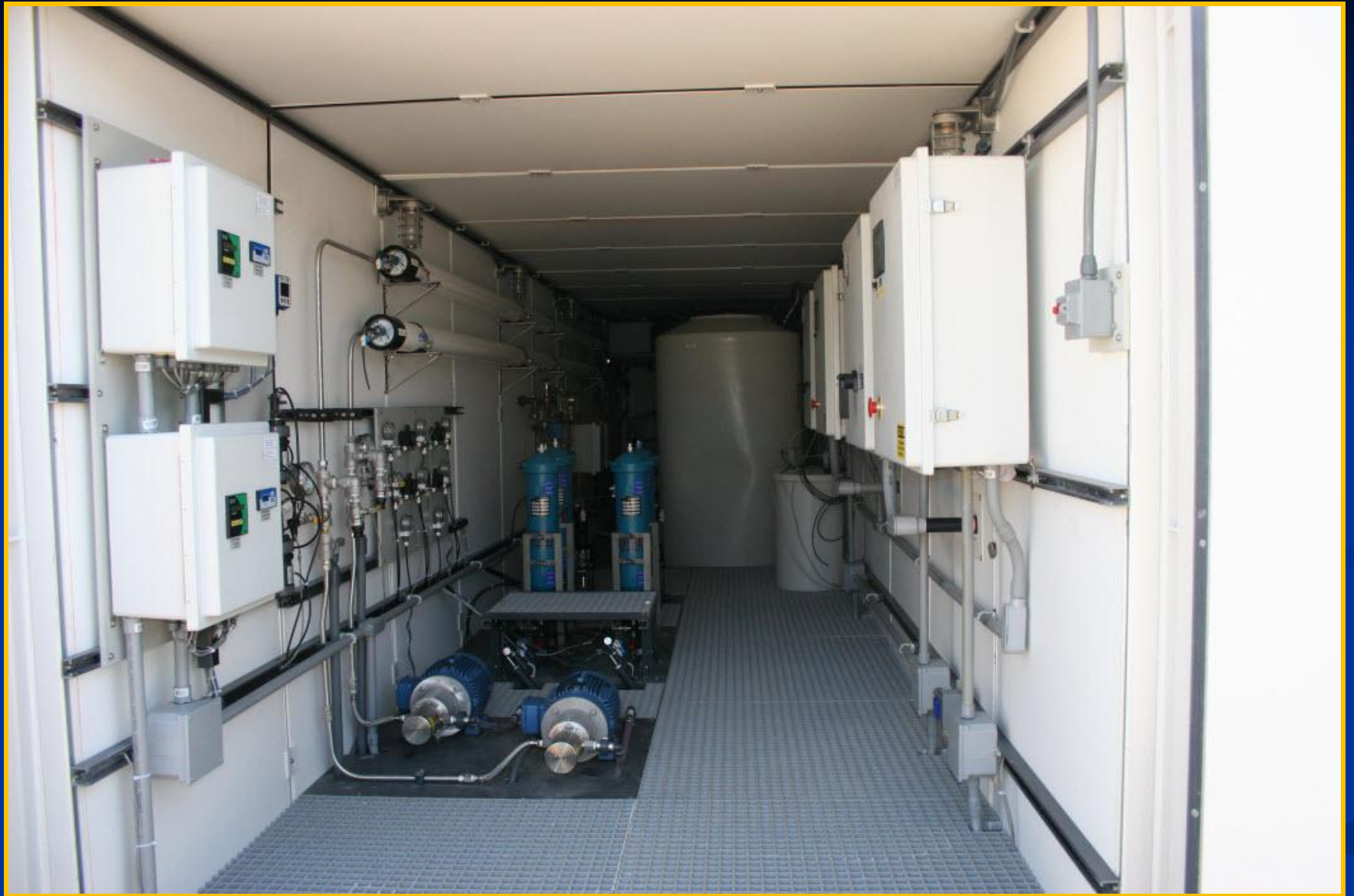
The Desalination RO system was comprised of Two (2) separate containers.
