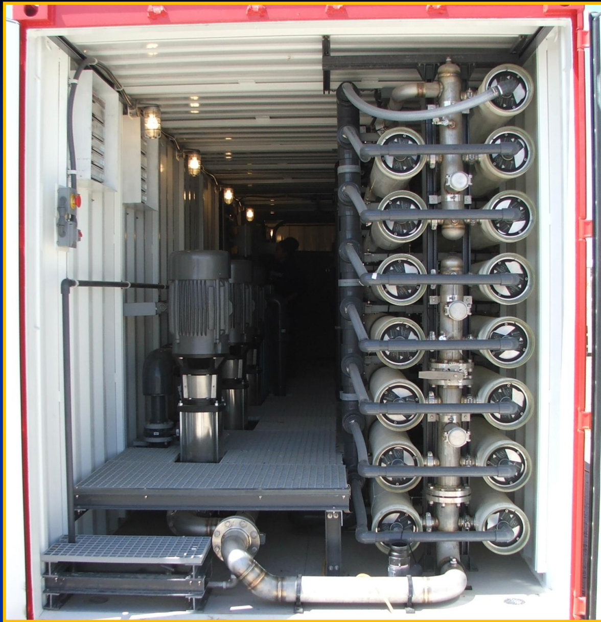
Each container housed a 500,000 GPD RO train.
