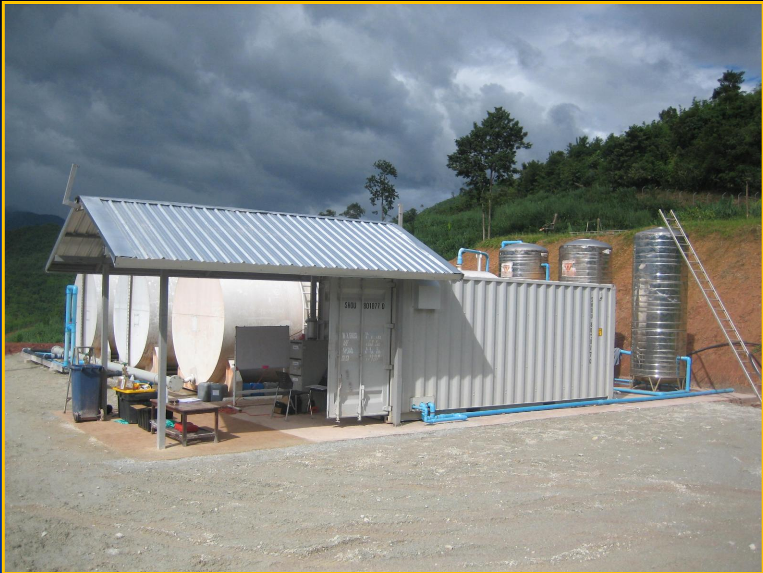
80,000 GPD Membrane Micro-Filtration System (MMFS) – This system is used for production of Potable Water from Raw River Water .
