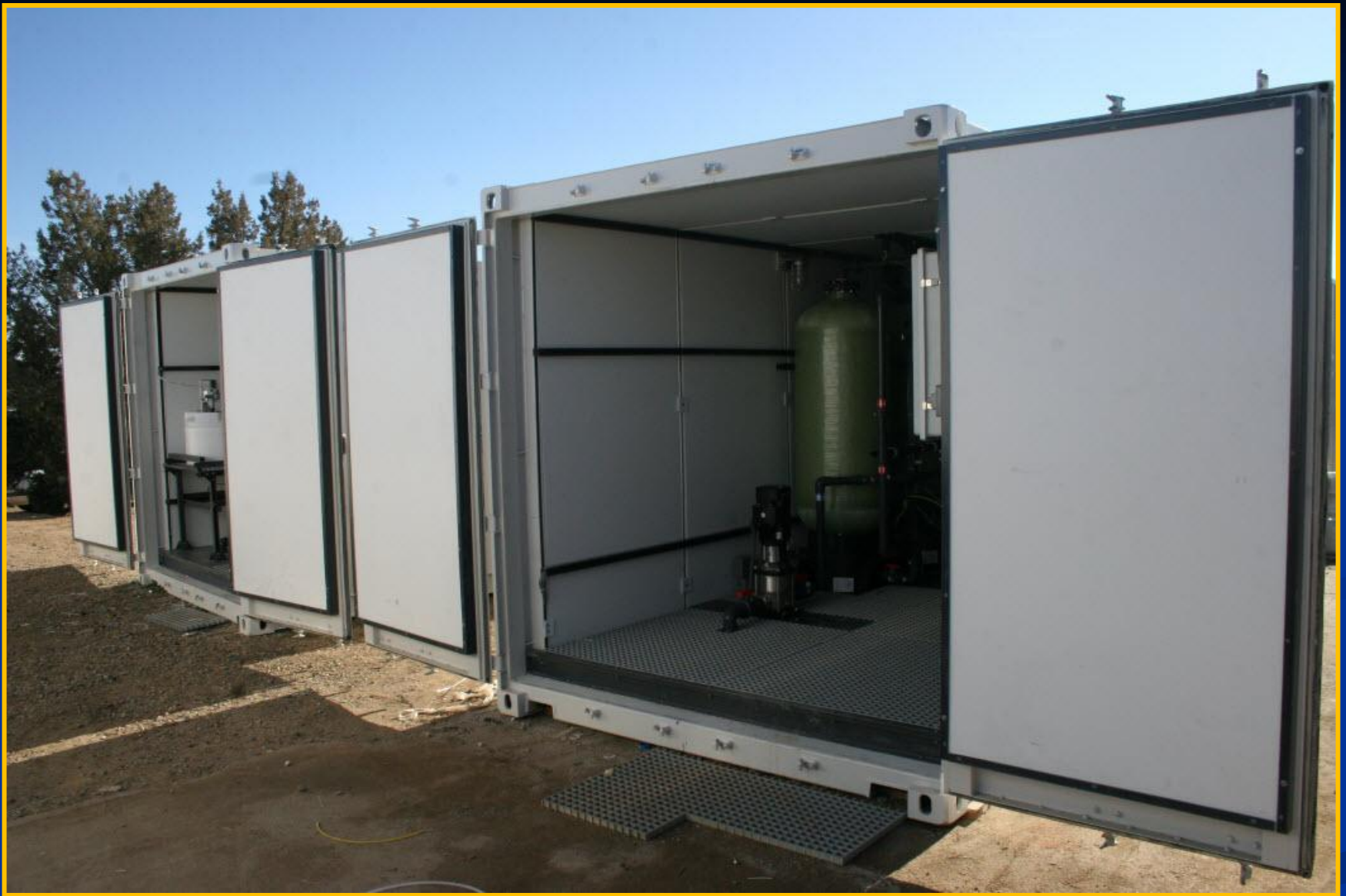
12,000 GPD Desalination - System is housed in three 40 ft intermodal shipping containers. Two (2) for Pre-Treatment, One (1) for the Reverse Osmosis (RO) system.
